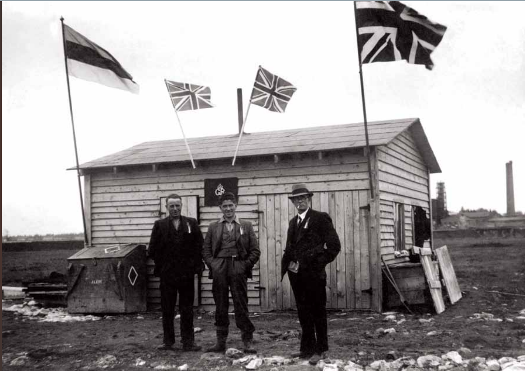
The work was supervised by the engineer H. M. Wallace, who had erected 15 radio towers before, with the actual assembly carried out by the Scottish technicians John Wallace and Alec Sutherland and Estonian workmen.
